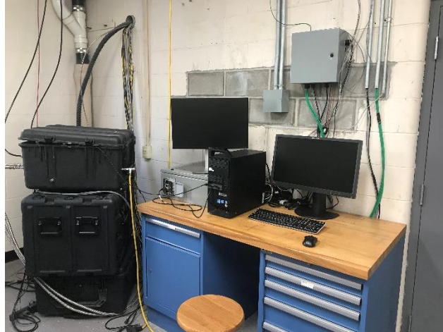
Figure 11: Continuous Engine Monitoring station with data acquisition and emissions equipment
