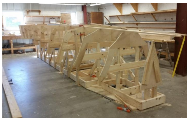
Figure 15: Construction jig for upper hull structure in place at The Landing School.
