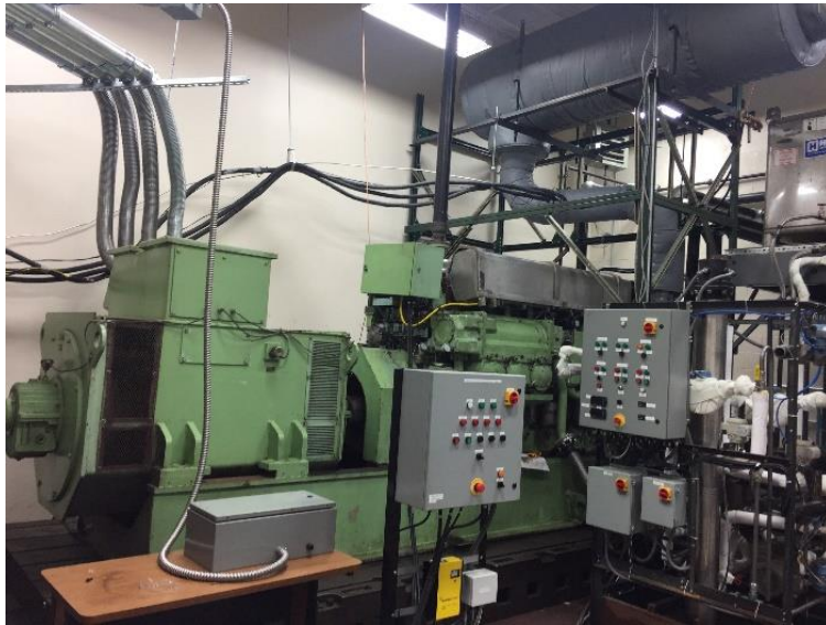
Figure 7: Photograph of installed medium-speed engine and ancillary equipment
