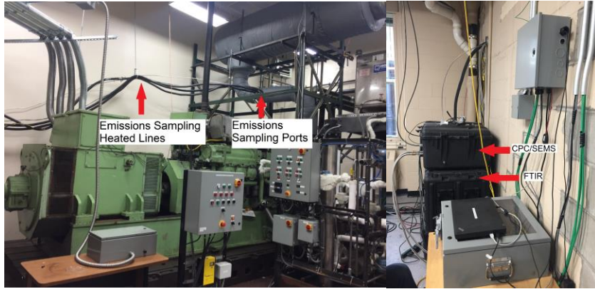
Figure 4: Continuous Emissions Monitoring system installed on Medium Speed Diesel
