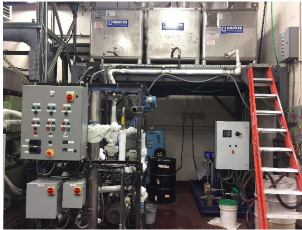
Figure 10: Fuel tankage mezzanine with fuel handling skid in the foreground
